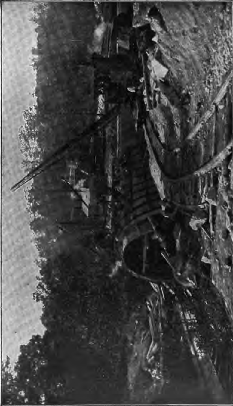
PLATE 145.—Contract 2. Cut-and-cover Aqueduct Building Plant. Stone crushed and concrete mixed at plant in distance. Concrete hauled in buckets to forms and placed by locomotive crane. Steel inside forms, outside forms of steel ribs and wooden lagging. First complete plant of this type.
